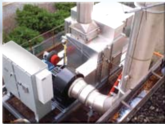
Waste Heat Recovery Achieved at Commercial Bread Bakery CatOx in Pennsylvania.
